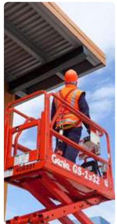
Figure 8: A worker restrained in scissor lift.
